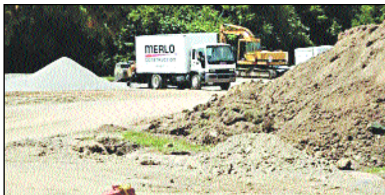
Work on the parking lot in McClumpha Park was halted by a stop work order issued by Wayne County last week.
